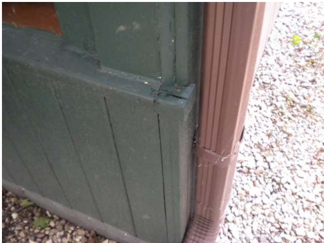
Rotted wood trim
