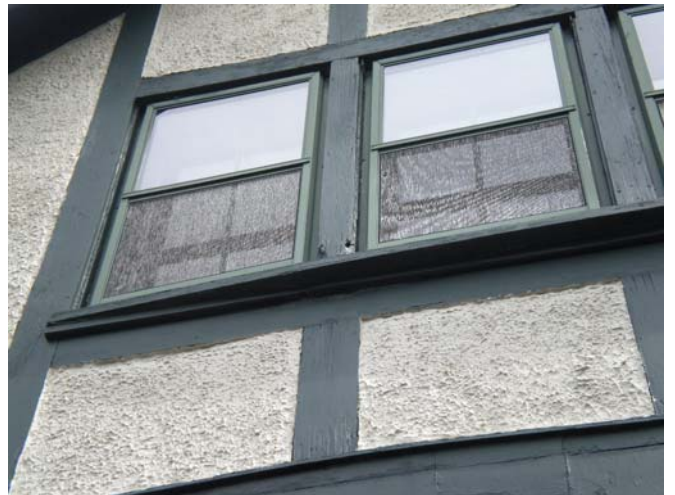
Rotted wood trim
