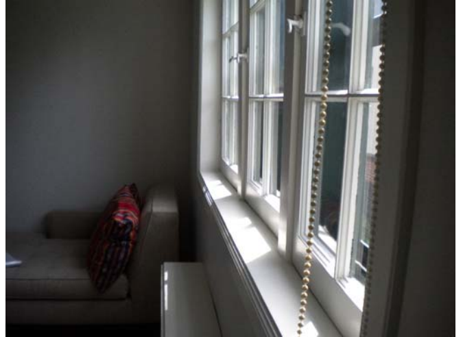
Wall out of plumb
