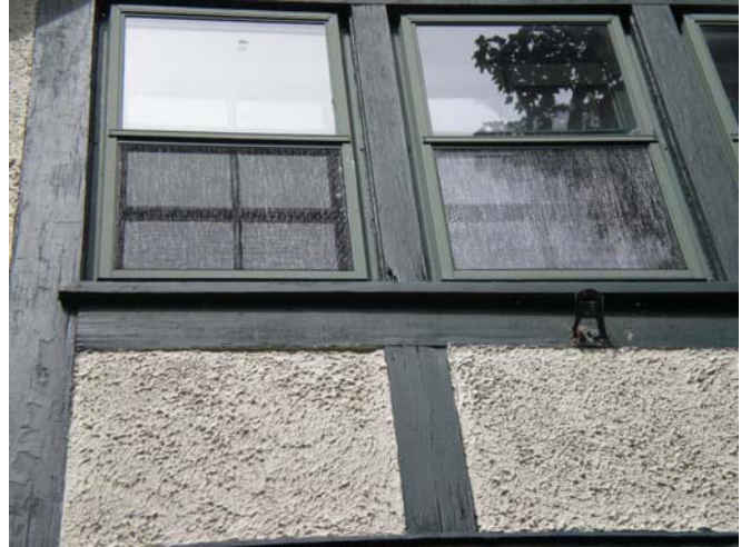
Rotted wood trim
