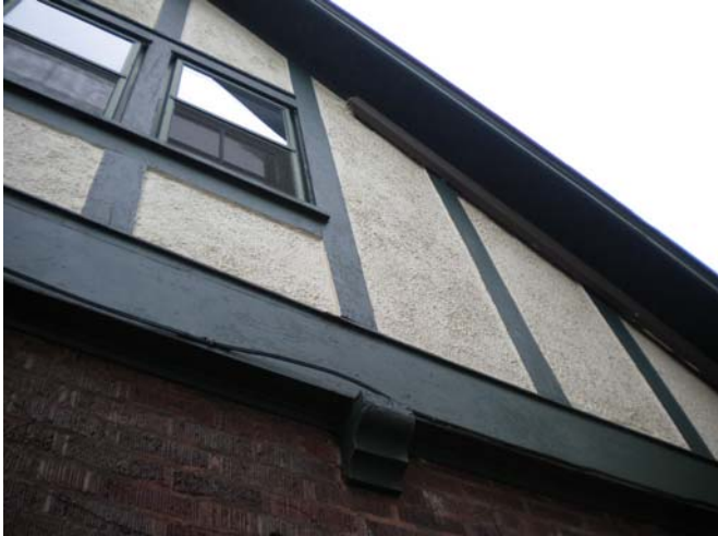
Rotted wood trim
