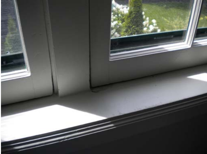
Staining on window
