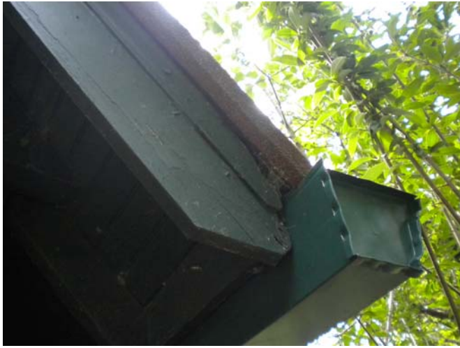
Rot at garage trim
