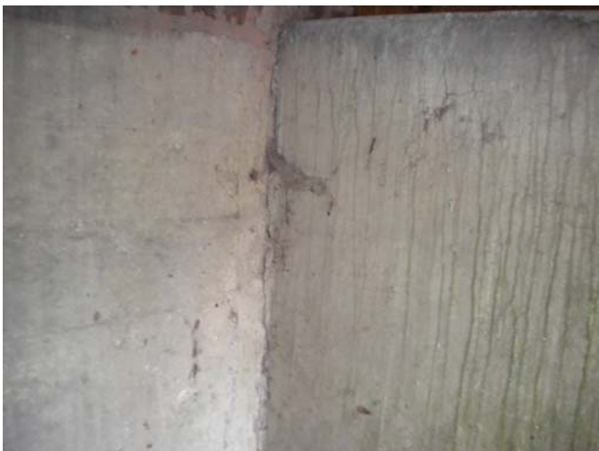
Cracking at stairwell
