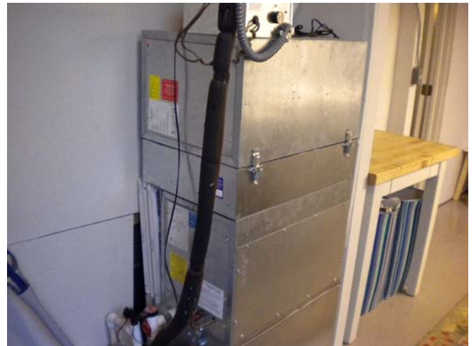
Basement air handler
