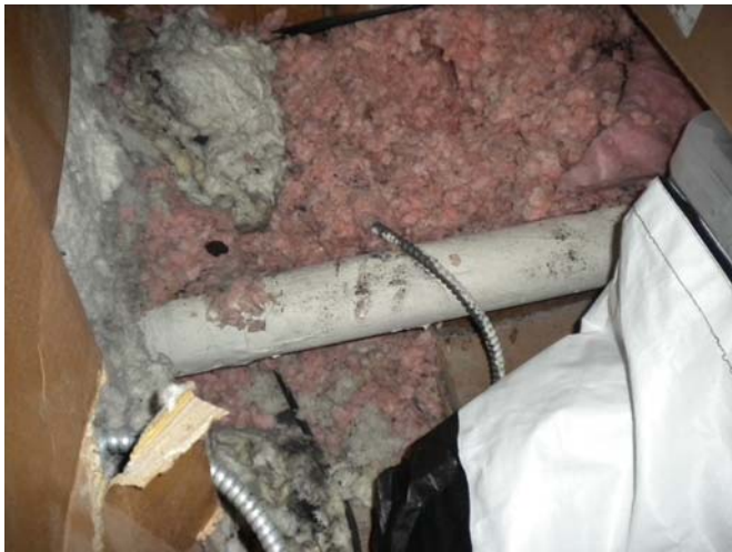
Possible asbestos material
