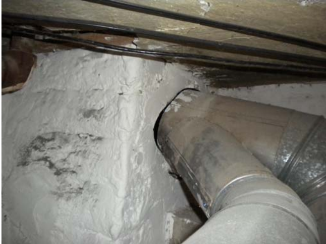
Flue gap at chimney
