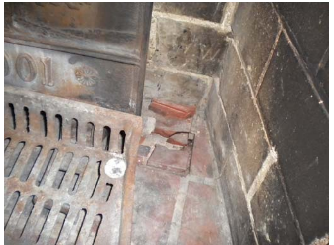
Damaged brick in fireplace
