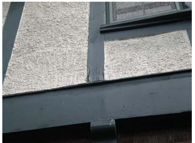
Rotted wood trim
