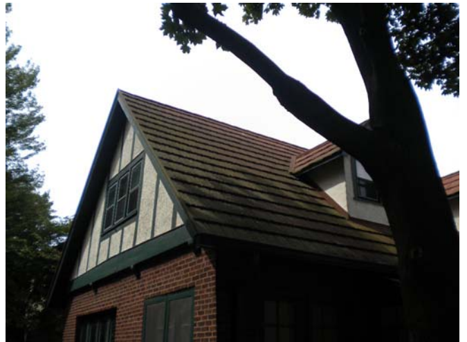
Moss on roof
