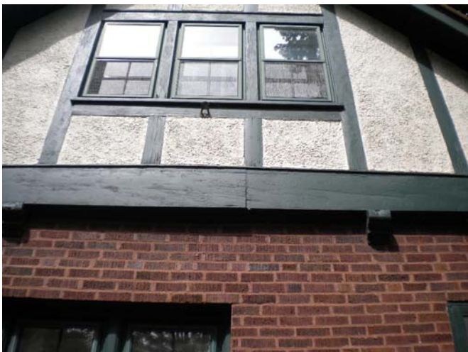
Rotted wood trim
