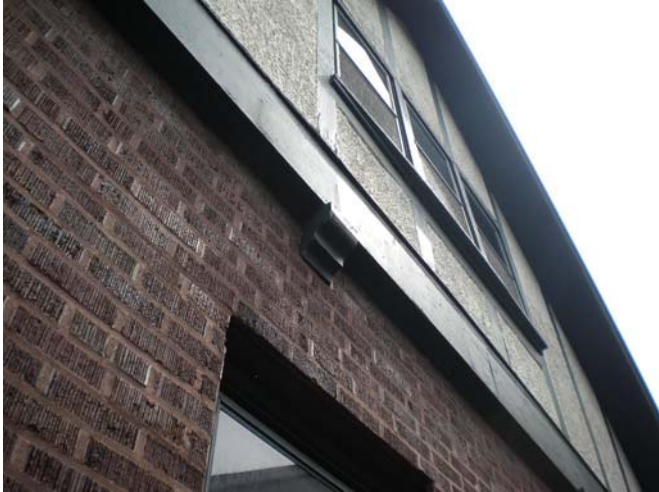
Deflection at west wall
