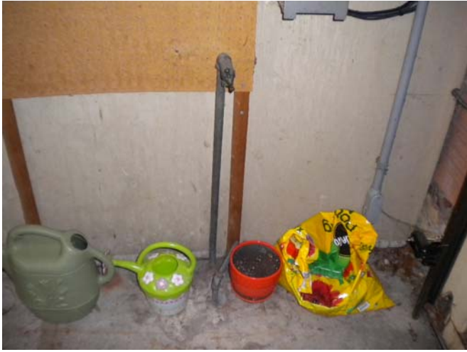
Abandoned piping in garage
