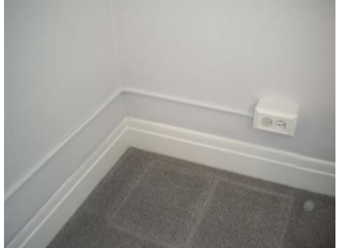
Exposed electric raceway
