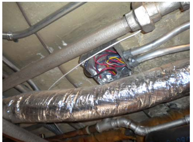
Open junction box
